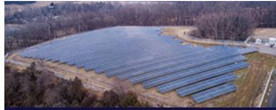
Mill Road - 18 MW
